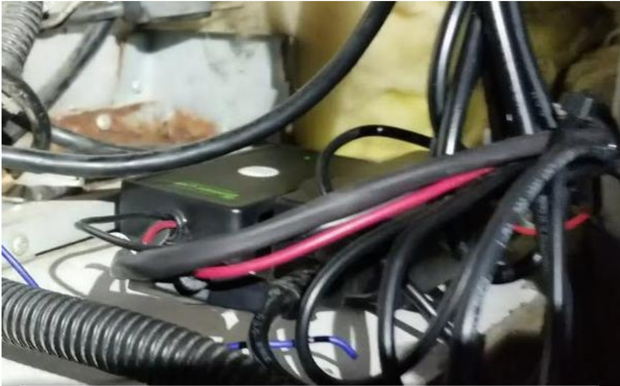
This is an example of the awning light LED controller being installed behind the refrigerator in this motorhome. The refrigerator was on the opposite side wall where the LED strip was mounted.
